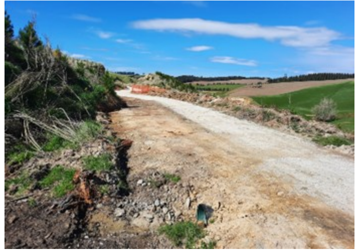
New track diversion around the major slip with additional culverts either end as a measure to reduce water flows in the vicinity of the slip
