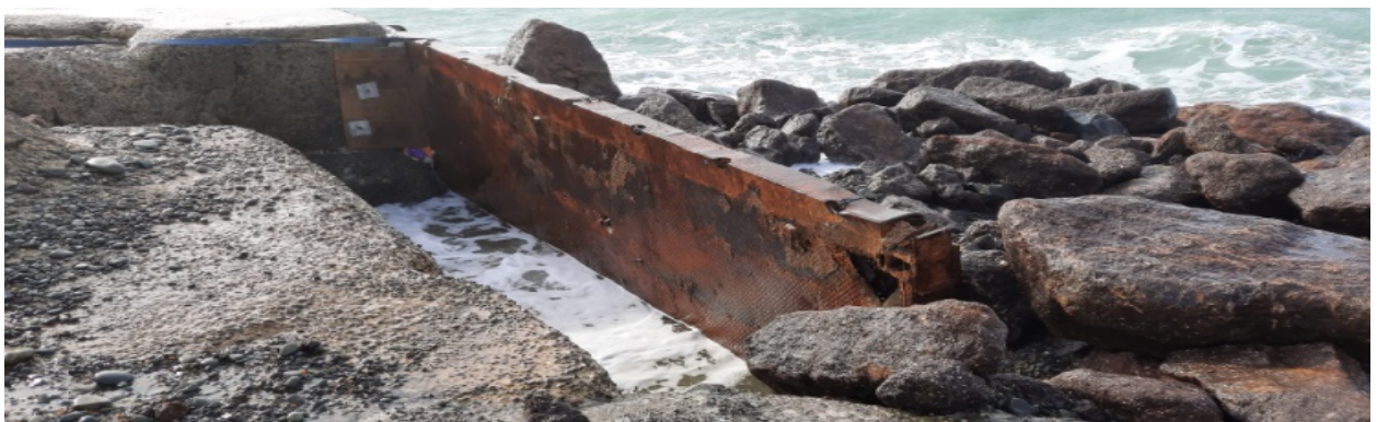
Railway carriage base (7m x 2.5m) formwork to eastern side of the breakwater head – ready for 25 cubic metre concrete pour to fill the large cavity
